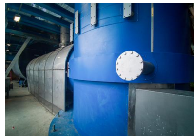
Figure 4: An installed steam boiler
